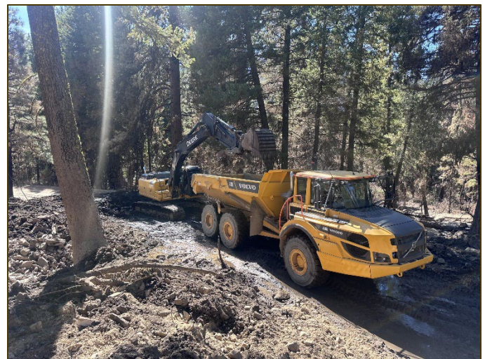
Figure 4 Debris flows from mid-September rains already impacted the Grandjean Road, causing fire crews to use heavy machinery to open the road for fire crews.
