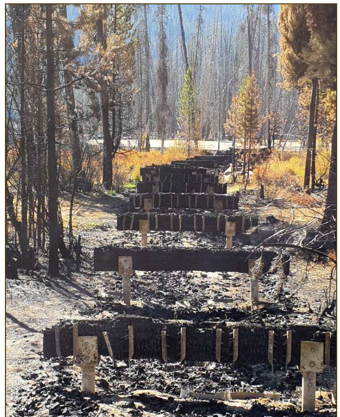
Figure 5 This popular boardwalk at Stanley Lake was destroyed.
